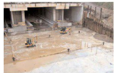
KTZ21.5 - well pots with submersible pumps
