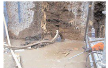
LB2-400 - minor dewatering when sealing the walls by means of small 1-phase submersible pump
