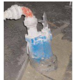
KTV2-37 flying pump in the area of the tunnel front
